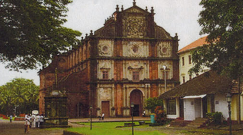
Lime plaster was stripped from the Basilica de Bom Jesus, leaving the stone exposed to the elements.
